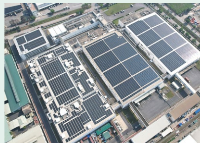
Solar power panels installed in fiscal 2022
