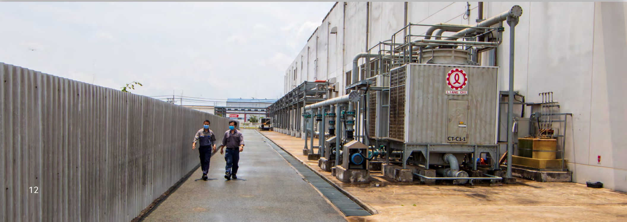
Water tank system at our Vietnam factory
